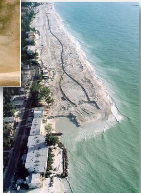
Figure 7.3: Beach nourishment by means of pumping sand onto the beach through a pipe system
